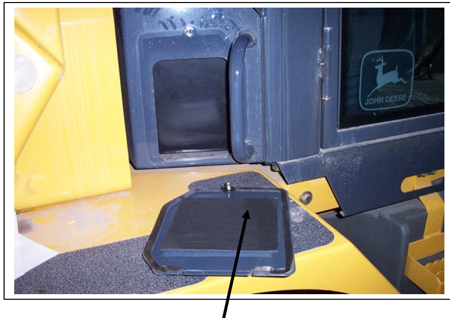
Outside air intake with louvers on door restricted by self adhesive foam panel
